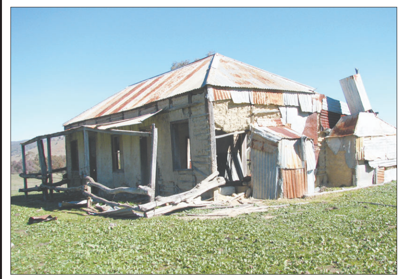
This deserted cottage has stood beside the Hargraves Road for as long as I can remember. Of wattle and daub construction, it has obviously been built by a craftsman, using round and adzed timber for the frame. It is sad to see something of heritage value slowly disintegrating until, in a few more years it will be no more. Peter Burns
